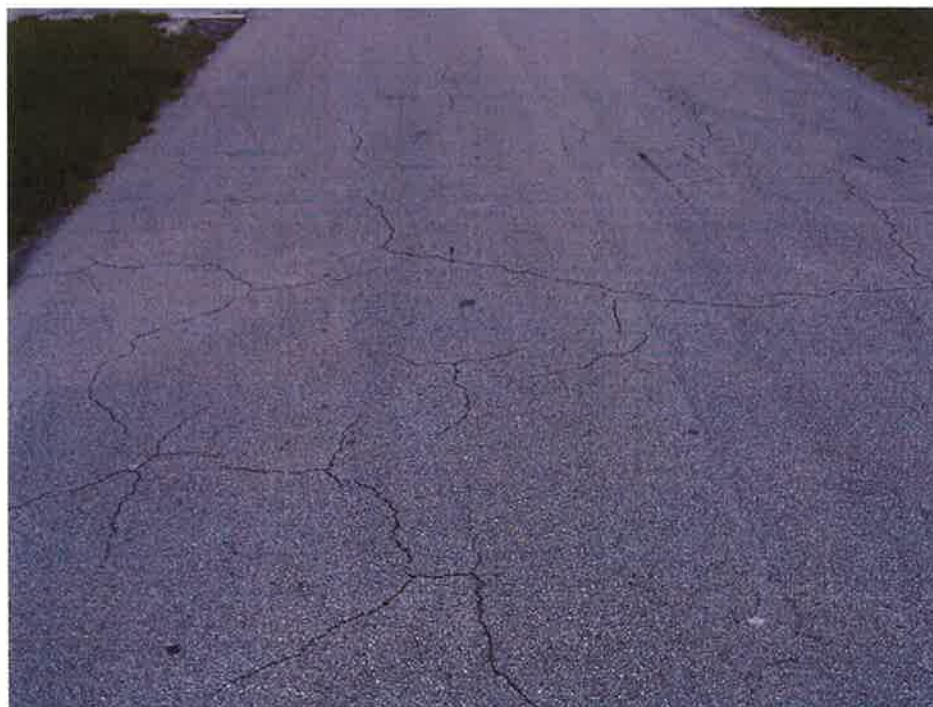
Picture 7: Alligator Cracks
