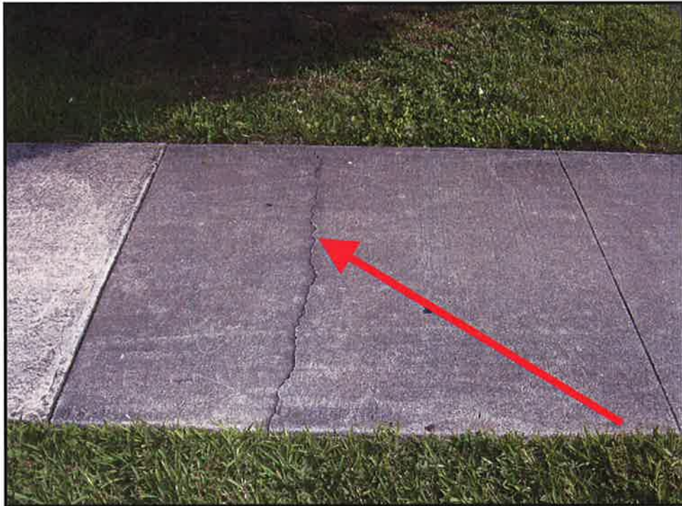
Picture 5: Typical Light Damage
