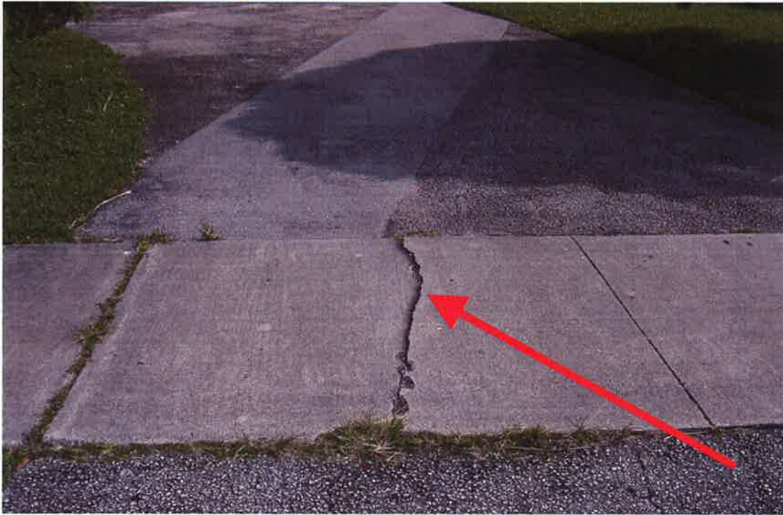
Picture 6: Typical Heavy Damage
